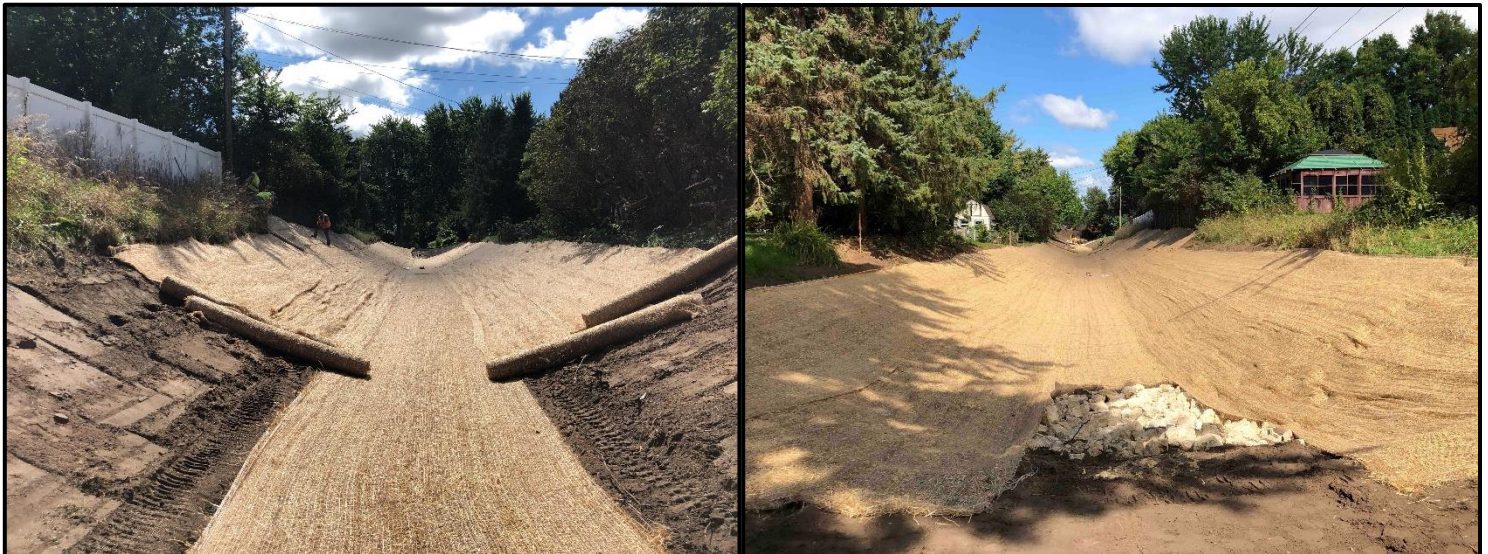
With the clearing and grading of the Louis-Ridge swale complete, crews seeded and installed biodegradable erosion control blanket
