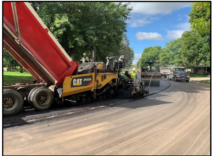
Paving of the final layer of asphalt in progress on Bohlken Drive
