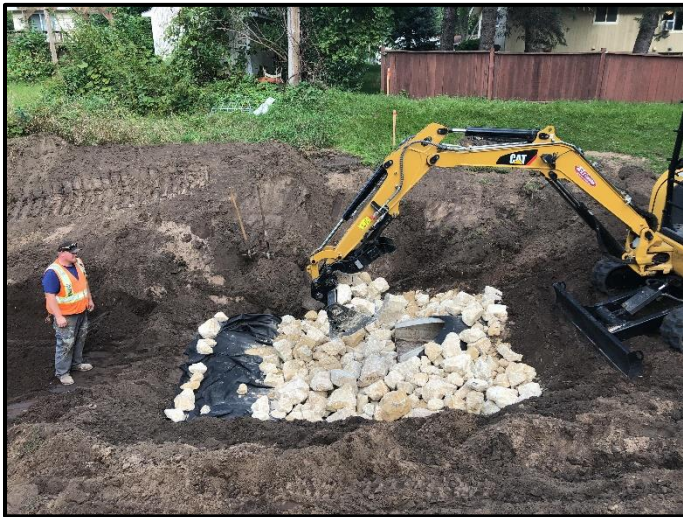
Installation of rip-rap rock around new drainage structures to reduce erosion is part of the grading and drainage improvements in the Louis- Ridge swale
