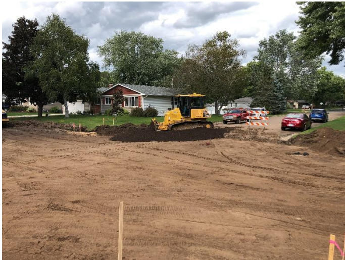
Placement of the base layer of gravel in the intersection of Manor Ln & 19 th St
