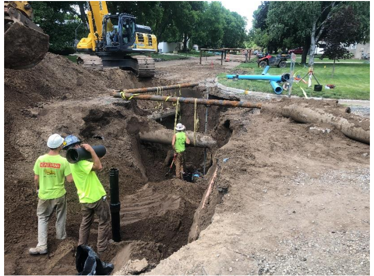
Existing storm sewer is supported with old water main pipe as new water main is installed below in the intersection of Manor Ln and 19 th St
