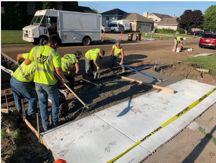
A replacement concrete driveway apron is poured next to a new section of sidewalk on 31 st St
