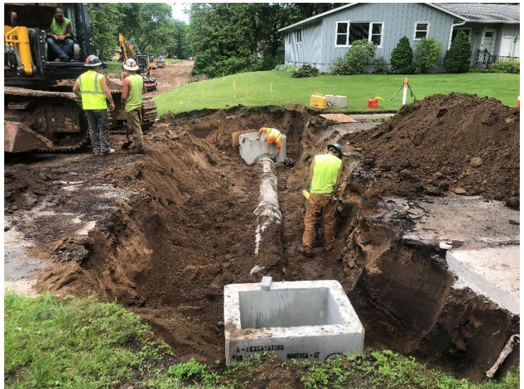
New storm sewer is installed across Louis Lane near 21 st Street Installation of new storm sewer will improve street drainage in the neighborhood.
