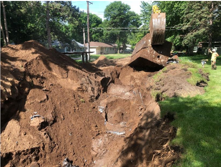
Removal of an old pressure valve vault near Pine St on 21 st St to make way for new water main
