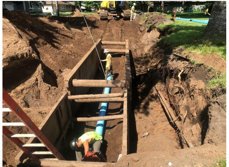
Gate valve replacement and water main installation near Pine St on 21 st St
