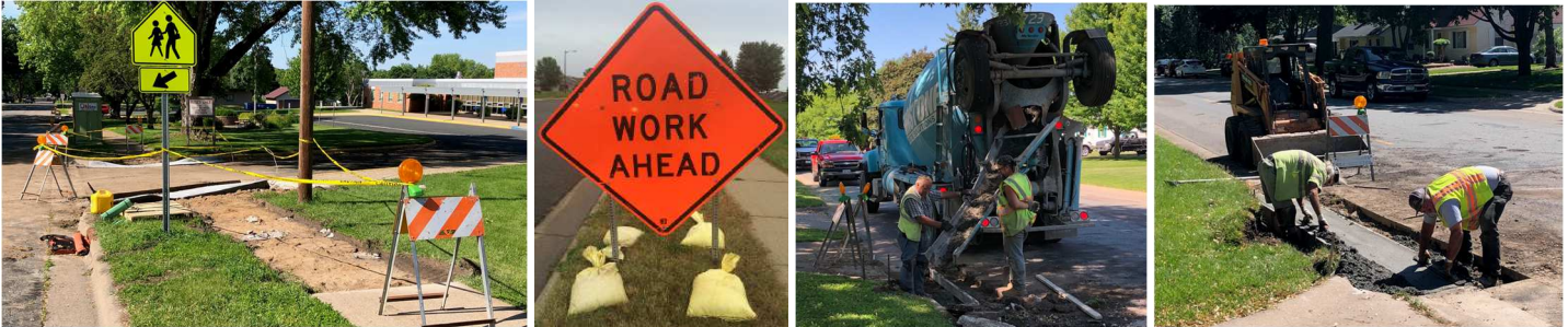
Above Left: Removing Existing Pedestrian Ramps....Above Left Center: Road Construction!...Above Right Center: Pouring Curb...Above Right: Finishing Poured Curb...
